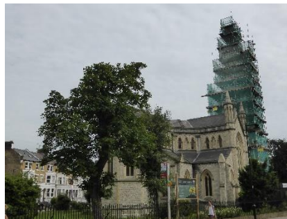
The spire is still fully clad in scaffolding and netting in July 2016
